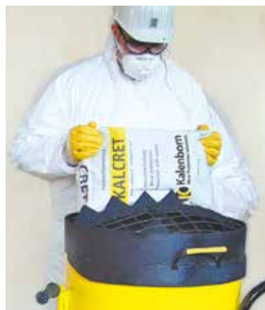
Material feeding into the forced circulation mixer
