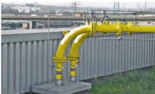
KALDETECT in a German waste incineration plant
