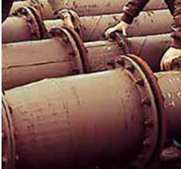
Expansion joint in a hydraulic ash line
