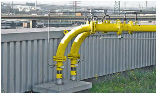
KALDETECT in a German waste incineration plant
