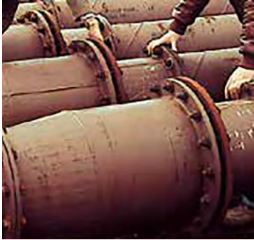
Expansion joint in a hydraulic ash line
