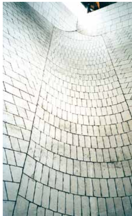
Bunkers for blast furnace charging are effectively lined with KALOCER
