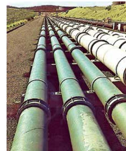
Wear protection for hydraulic and pneumatic pipes
